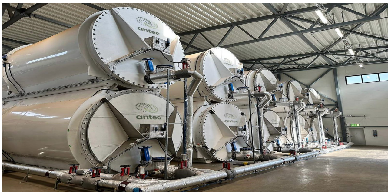
Plate 2: Typical Reactor Bank
